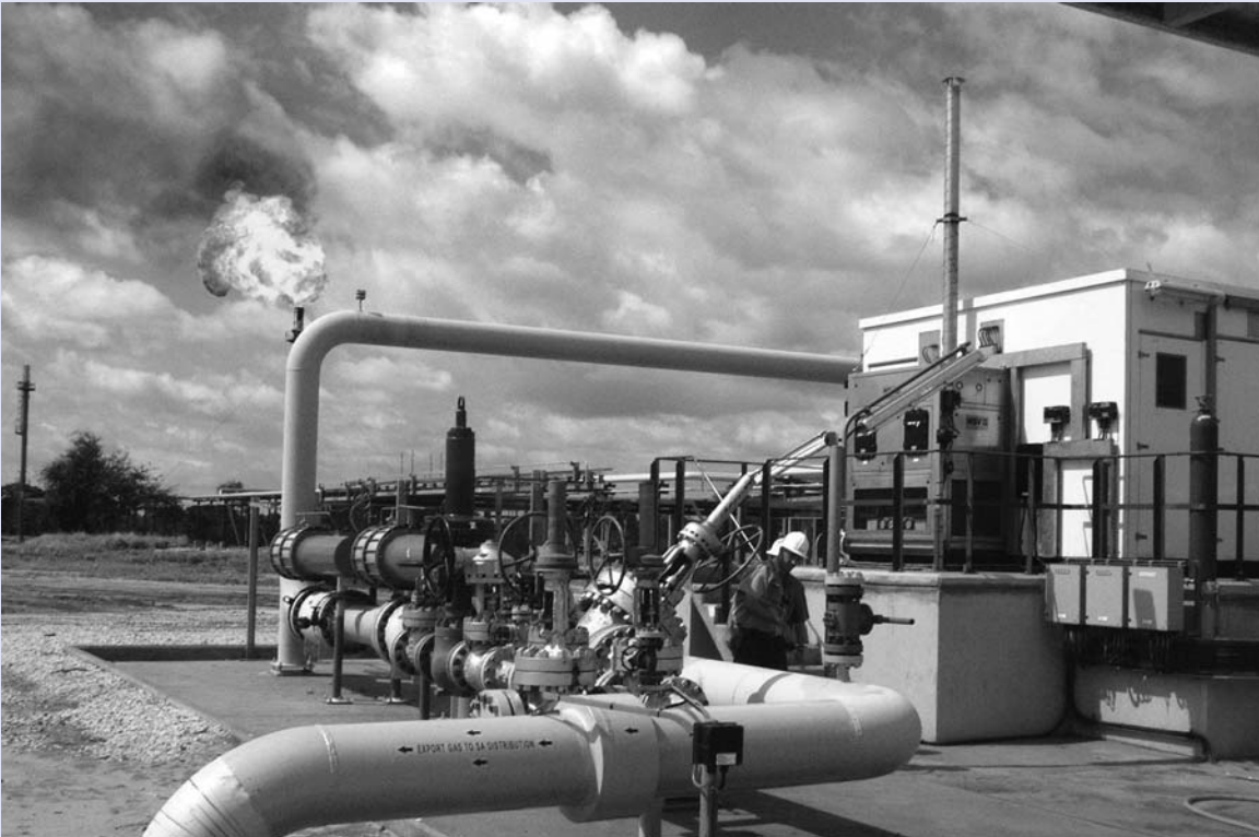
Gas flaring and pipeline equipment, SASOL Pipeline, Sub-Saharan Africa. Photo courtesy of SASOL/IFC.
