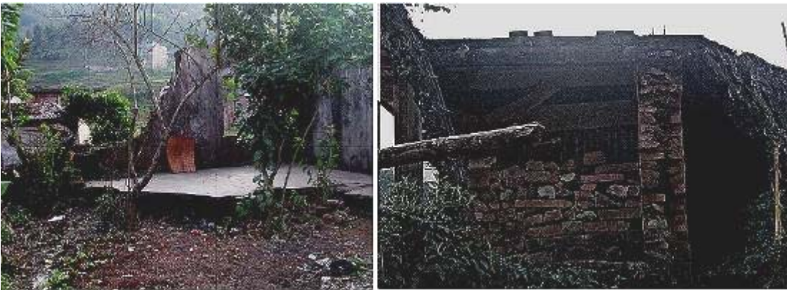
Figure 5.16. A section of the left bank of Araundi that suffered huge losses during the 1998 floods.
