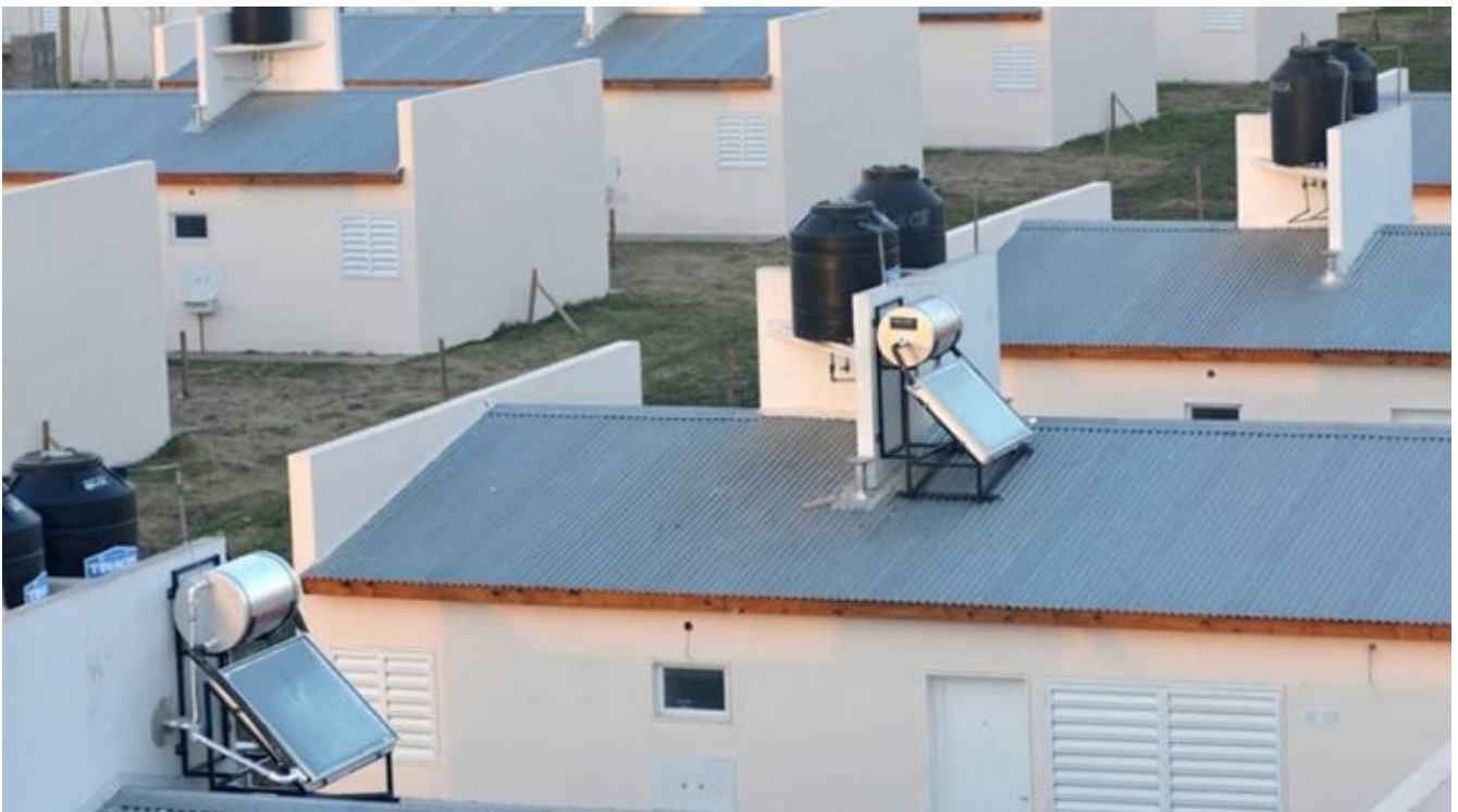
Solar Panels in Barrio La Perla. (Source: http://cedu.com.ar/ )
