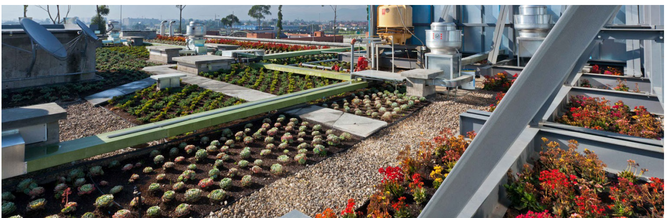
Green cover Alloat Bogota Airport, one of the hotels in Colombia with LEED Leadership in Energy and Environmental Design. (Source: coronamejoratuvida.com)
