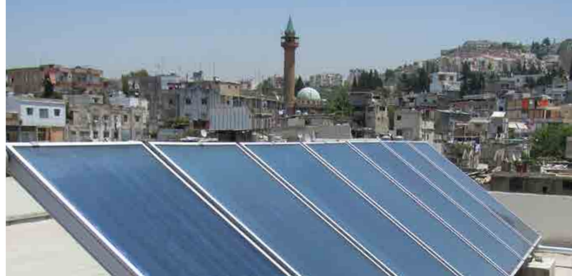
Solar water heaters, Saïda Government Hospital, Lebanon
