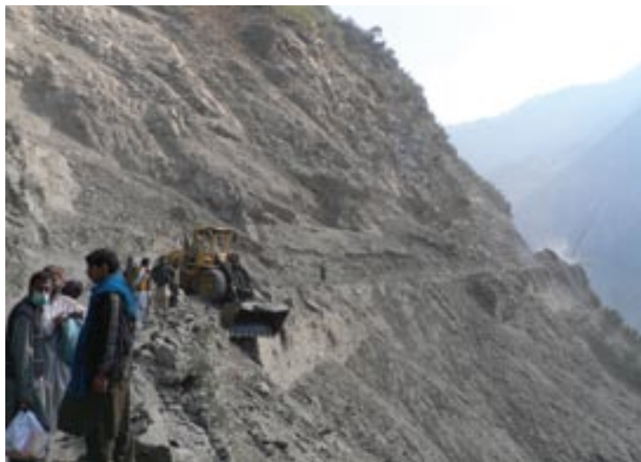
The danger of landslides severely hampered the relief effort until the advice of a slope-stability expert was secured
