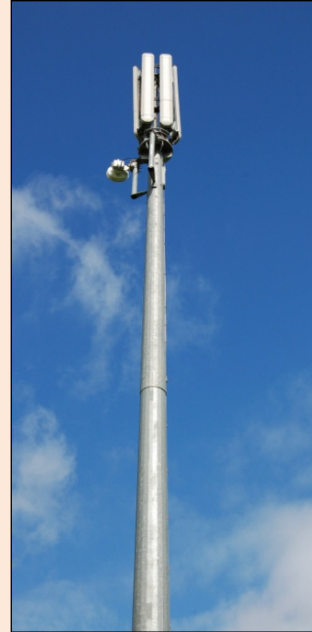
Figure 10. Mast and antenna sharing.
