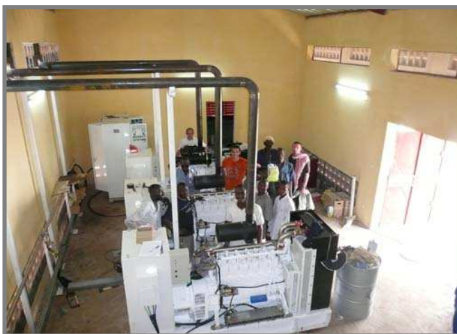
Three generators at Garalo
