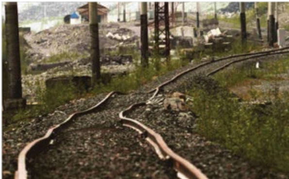
Fig. 2.8.8. A section of railway track damaged by permafrost effects.
