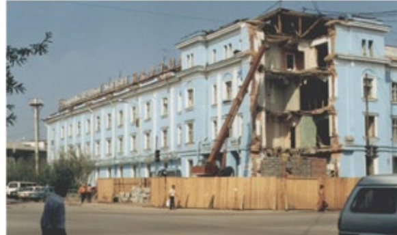
Fig. 2.8.11. The collapsed corner of a building in Yakutsk (Russia).
